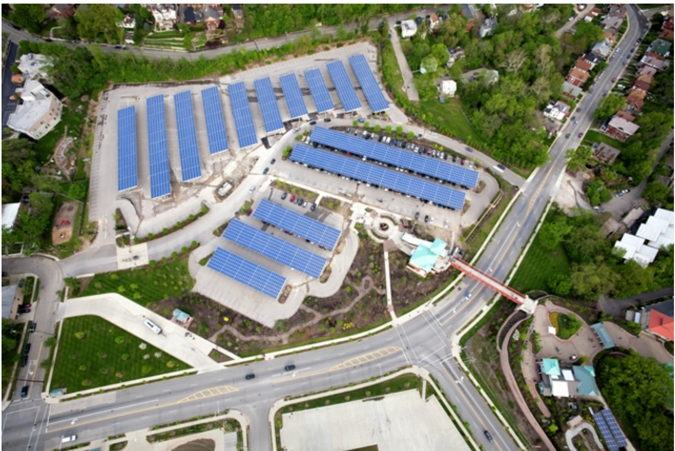
Parking lot 1.56 MW solar canopy
