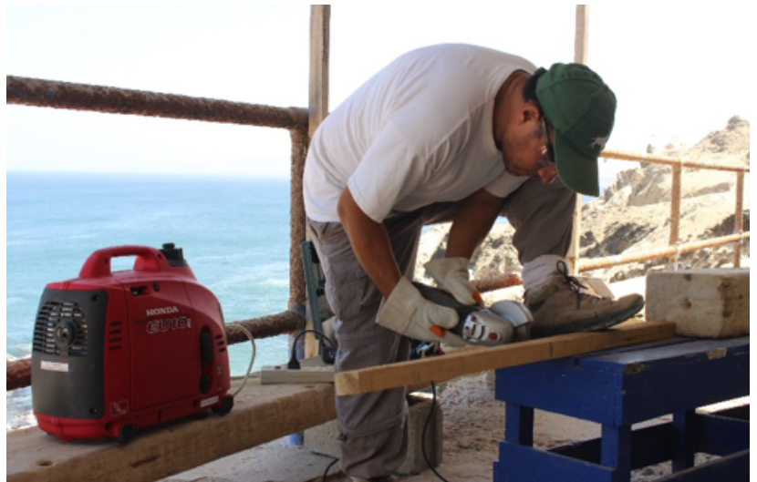
Punta San Juan Field Coordinator Marco Cardeña uses the power generator and tools to construct a wooden structure to mount time lapse cameras that will be used in the field for wildlife monitoring
