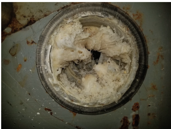
Severely clogged plate
